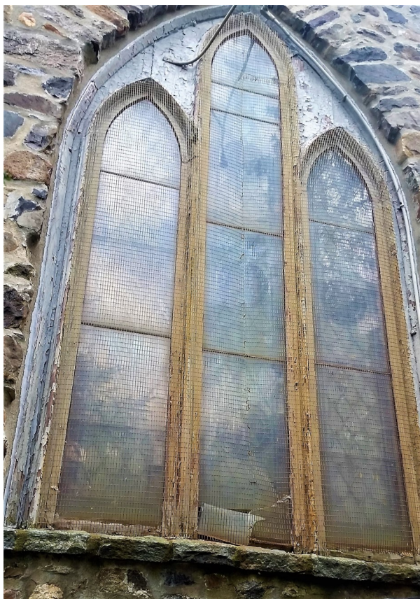
Ongoing deterioration of church windows is becoming an urgent problem.
